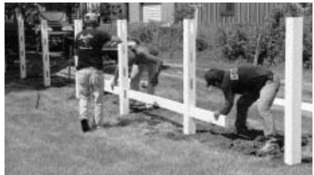
Threading the first rails, starting at the bottom. If spacing permits, rails are staggered at the joints.
