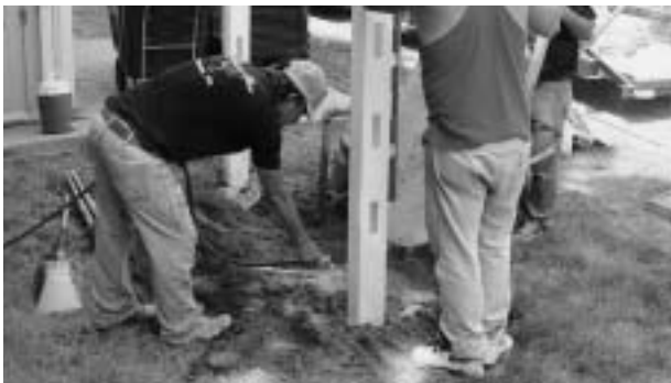
Holes dug, posts aligned and initially tamped in dry cement, water is being added to set the posts.
