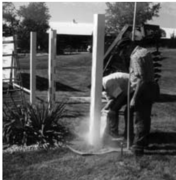
Once the post is aligned, cement or a cement-water mix will make it permanent.
