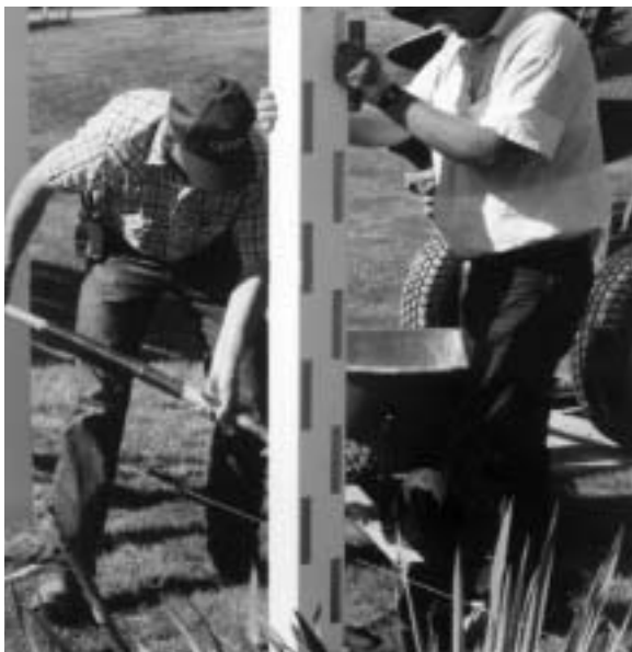
Post placement is important, using a stringline and level to assure vertical alignment.
